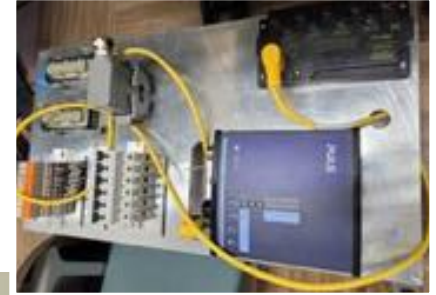
redesigned PLC automation
