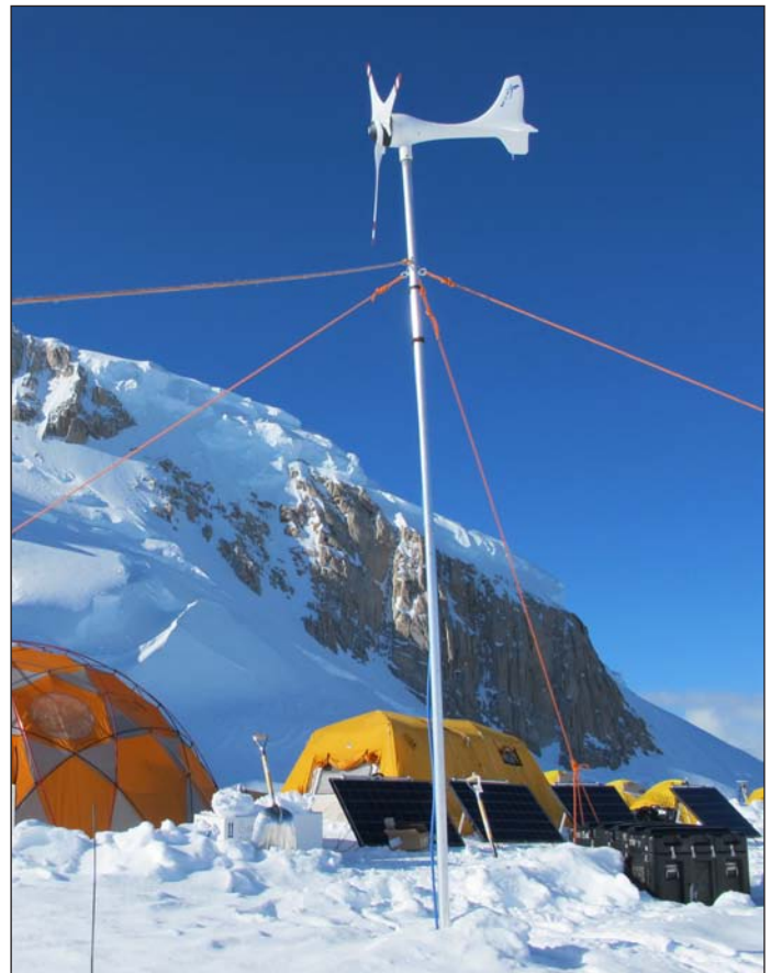
New solar and wind power system used for Badger-Eclipse drilling in Denali National Park. Photo: Mike Waszkiewicz
