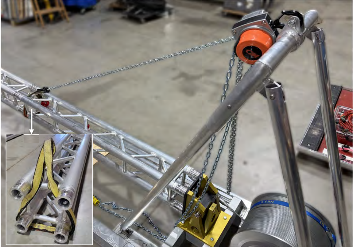
Figure 12-2: Chain hoist connected to the lifting frame and tower. The inset picture shows proper routing of the web strap on the tower truss.
