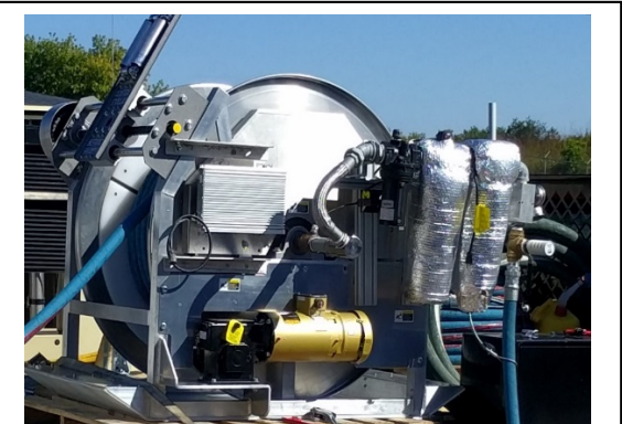
Fig. 5: Air Treatment and Hose Reel.
