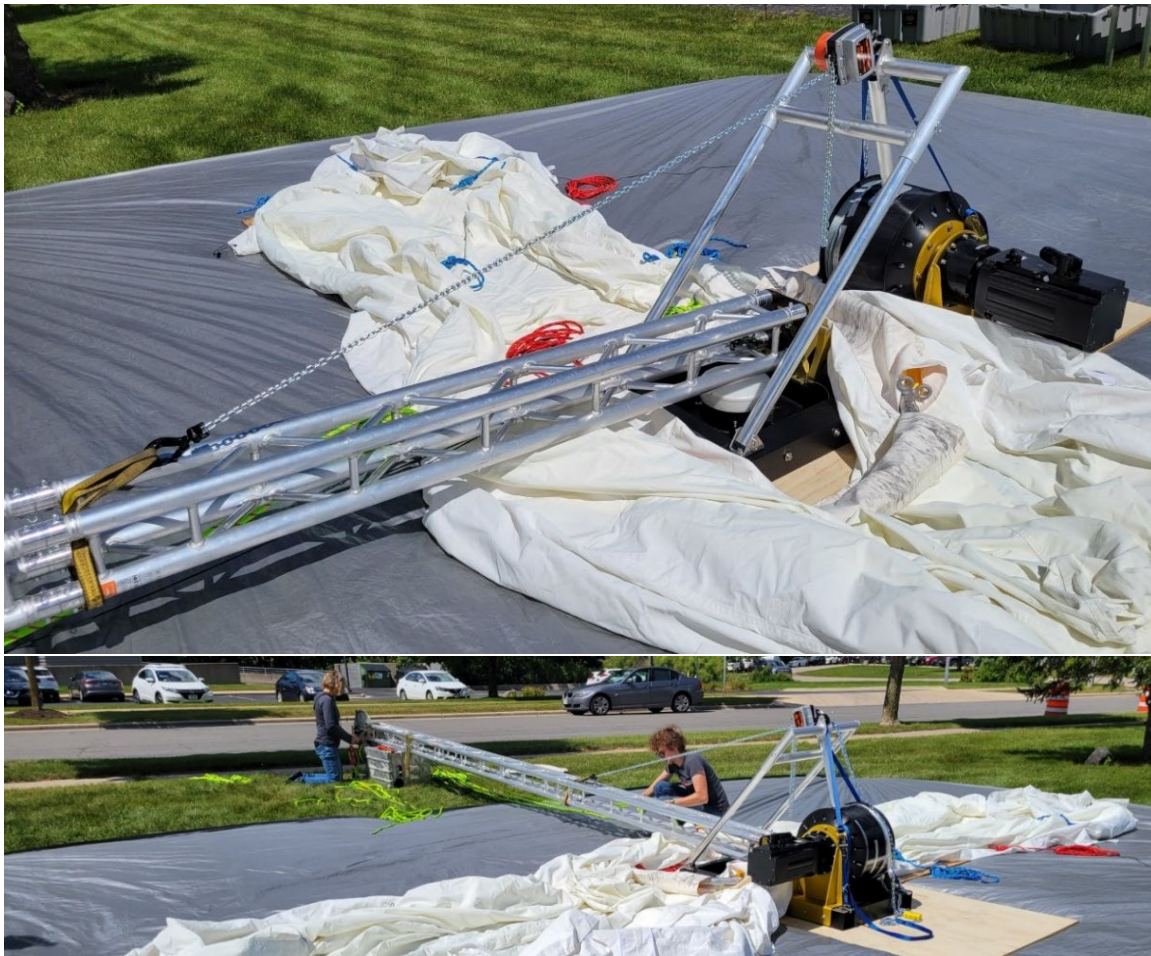
Figure 25: Tower lifting components installed on the winch base and connected to the tower.
