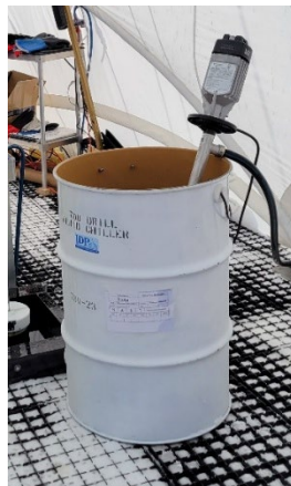
Figure 17. Lutz drum pump being used to transfer fluid back into drums after the fluid was bailed from the borehole.
