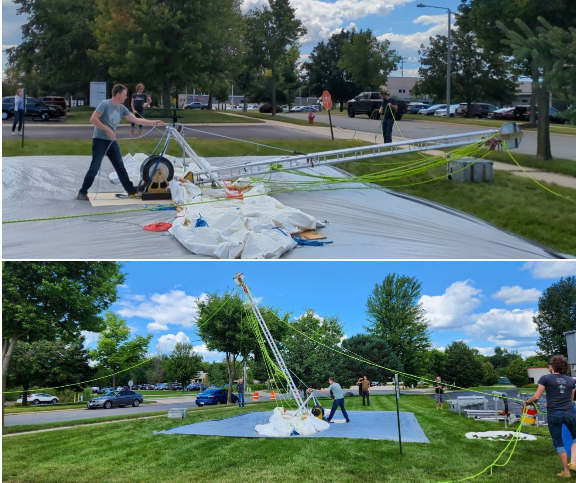
Figure 26. Raising the tower using the tower lifting fixture and team of people.
