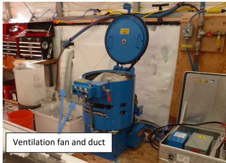
Figure 28. Centrifuge/Chip Melter ventilation
