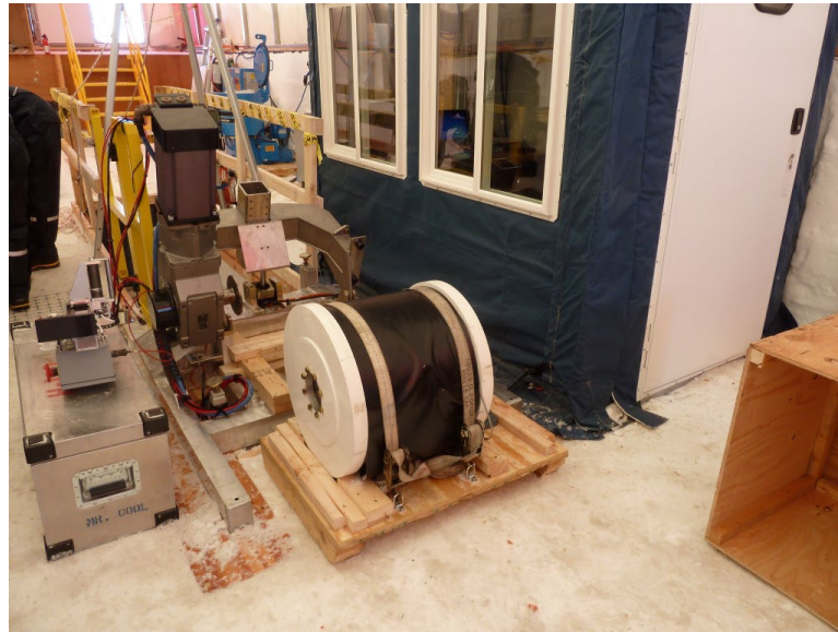
Figure 18. Tower base and winch drum
