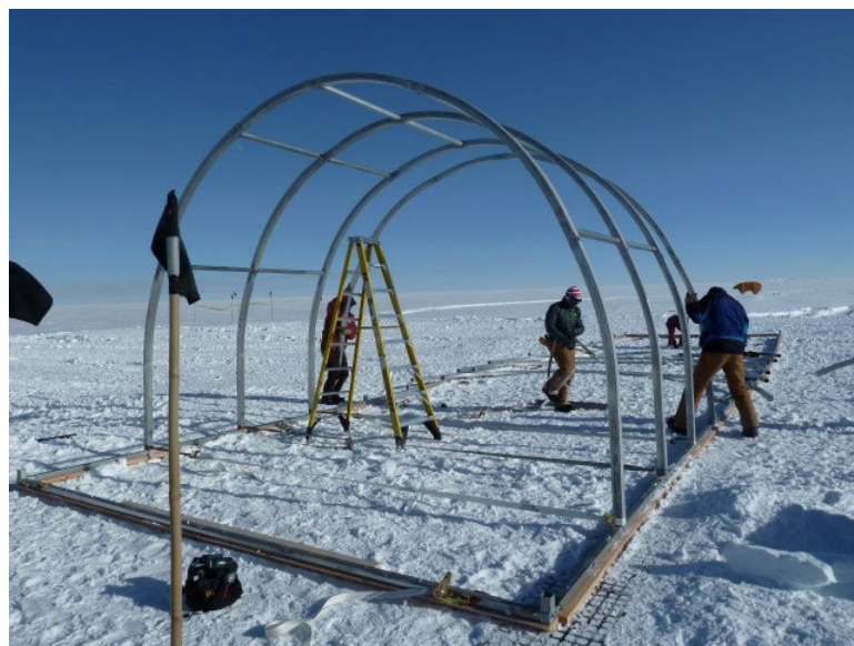
Figure 6. Tent frame being assembled off the end of the trench on the Geoblock footer tails.
