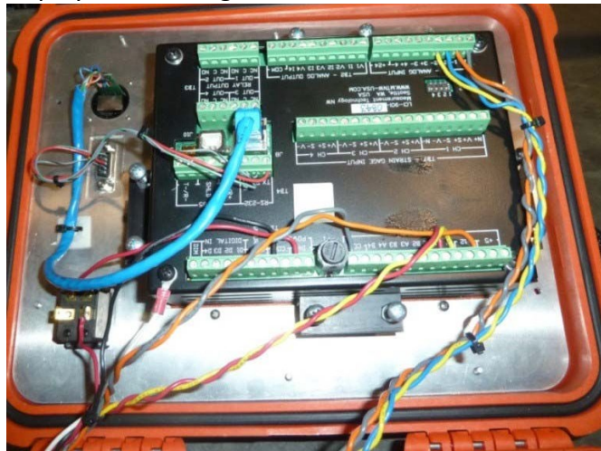
Figure 5: Pelican display case wiring
