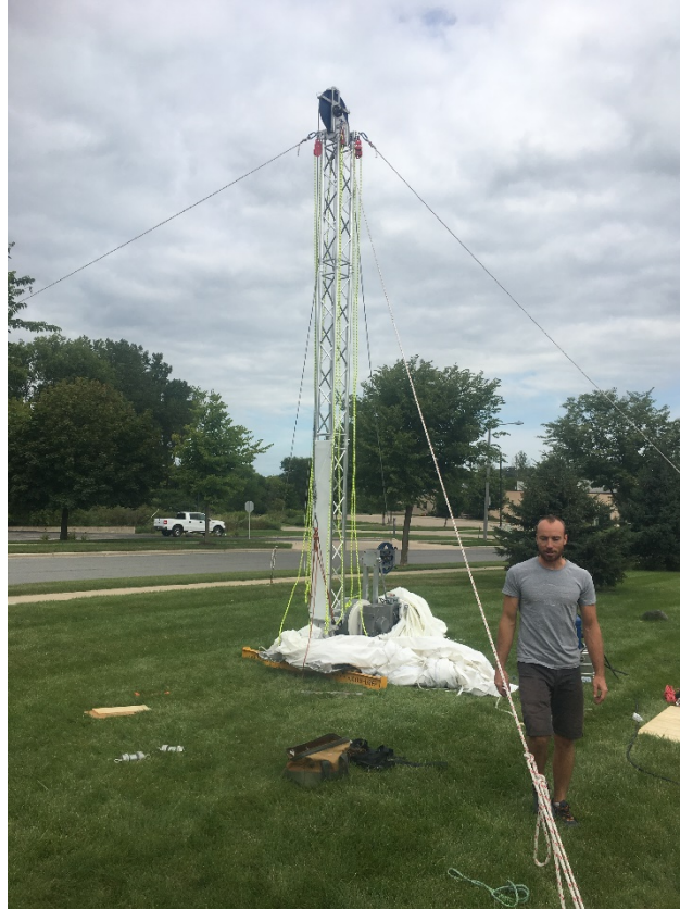
Figure 12: Secure 4 guy lines at 20' from bore hole with anchors appropriate for surface conditions.
