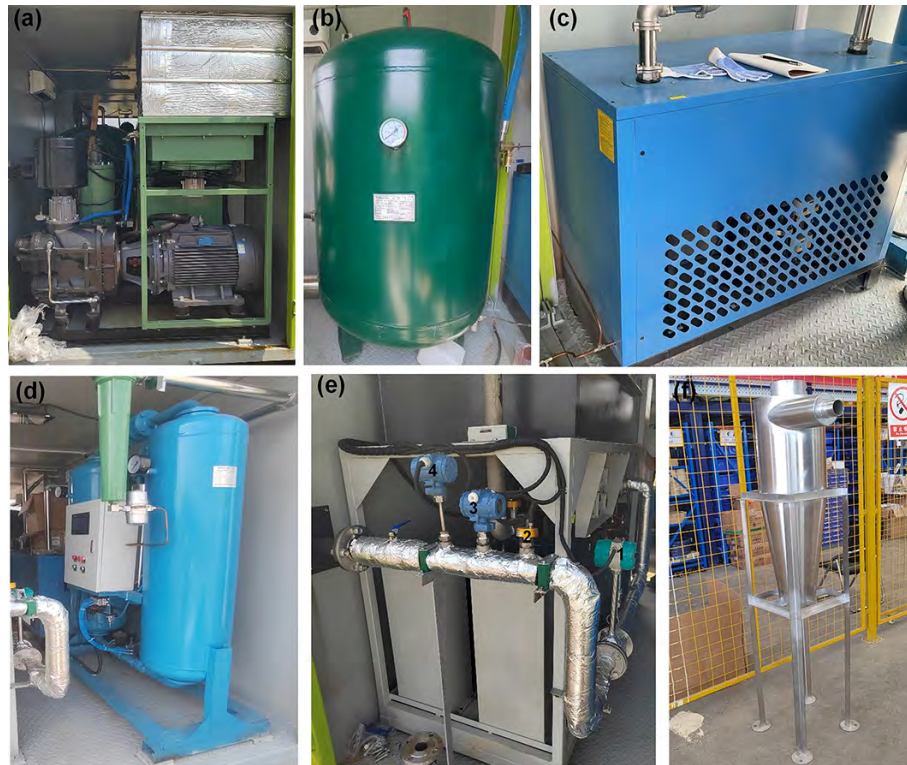
Figure 3. Main components of the air system: (a) air compressor; (b) air receiver; (c) freezing dryer; (d) desiccant dryer; (e) air cooler, 1-flowmeter, 2-dew-point hygrometer, 3-manometer, 4-temperature sensor; and (f) cyclone dust collector.
