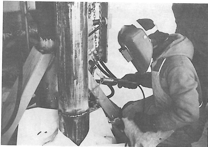
Fig. B-12. Each casing length had to have a continuous weld at each end. Note asbestos blanket around casing.
