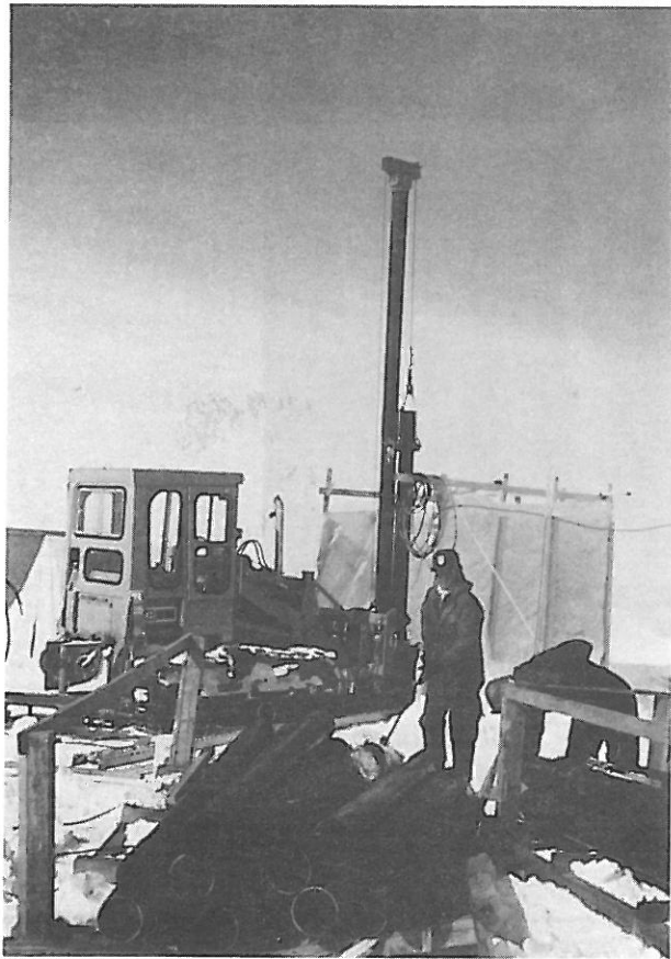
Fig. B-13. Prior to raising the casing into position each pipe was cleaned as thoroughly as possible.
