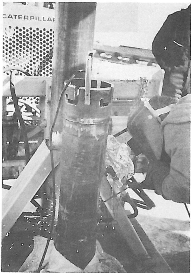
Fig. B-14 Because of the Danish winch design, the top 30 ft of casing had to be removed after freeze-in. A special adapter allowed the top lengths to be separated from the rest of the casing.
