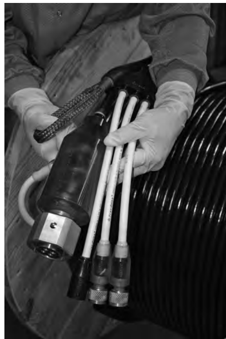
Fig. 7. Detail of the return water pump and instrumentation cable termination.
