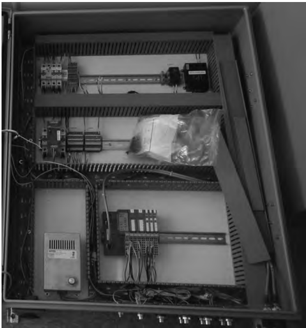
Fig. 6. IO panel partially constructed (UPS has yet to be installed at top).
